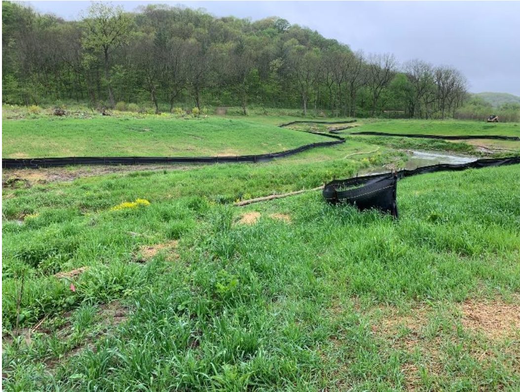
May 2020 photo of Mill Creek at Big Mill Wildlife Management Area, Jackson County, Iowa. Floodplain excavation, seeding, mulching, and silt fence installation complete for Phase II of floodplain restoration.
